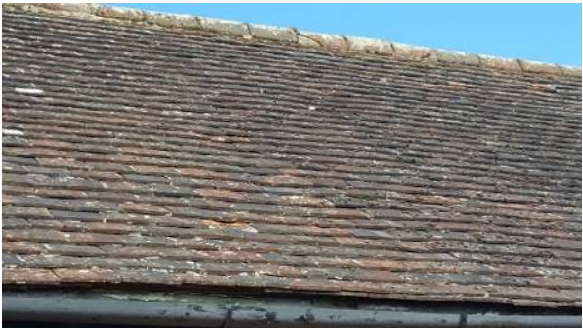
Plate 9: Showing raised roofing tile which shows potential bat access.
